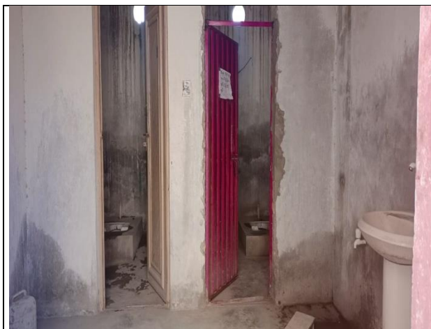
Washrooms in unhygienic conditions
