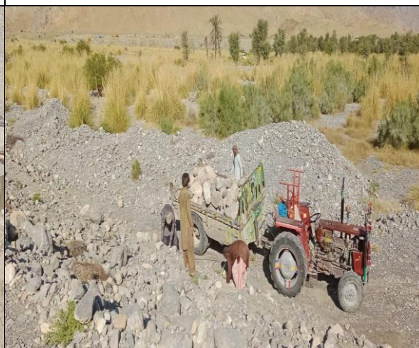
Workers without PPE's.
