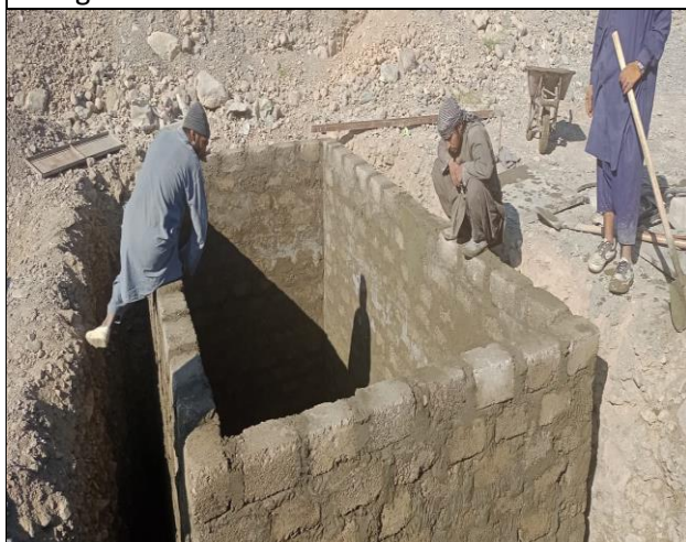
Site workers working without PPE's.
