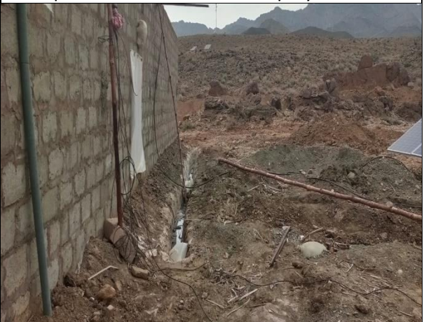
Open drain needs to be covered in proper pipes & barricading around campsite is required.
