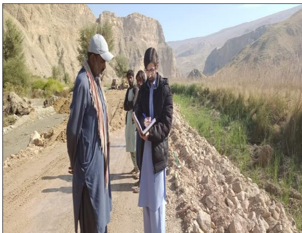
SC environmental specialist discussion with site supervisor to provide complete set of PPE's.
