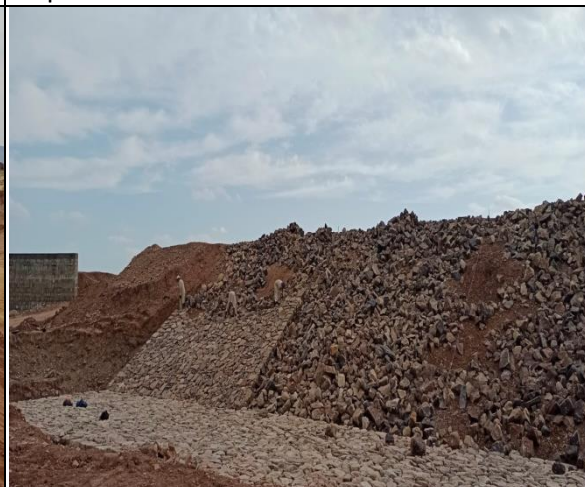
Workers not willing to wear PPE's.
