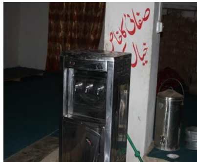
Figure 21: Hot /Cold Water Cooler
