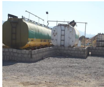
Figure 35: On-site Petrol pumping station
