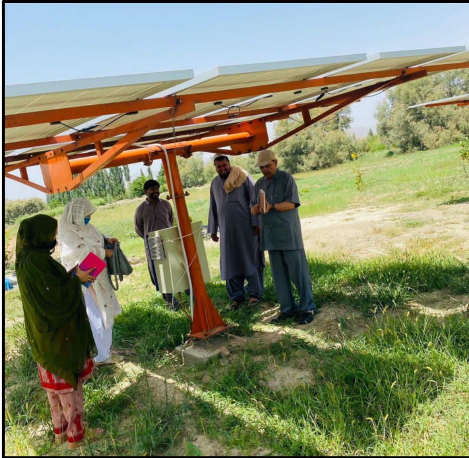
Figure 10: Visit Solar power System Installed at Village Badenzai Zhob
