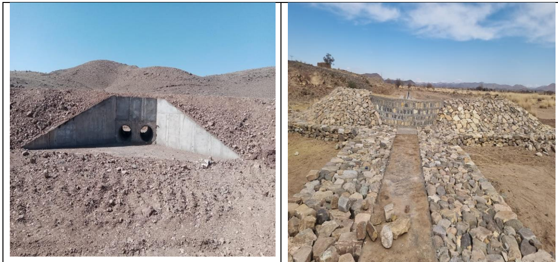
Local community demanded to provide additional culvert which was logical to construct at the above mentioned RDs to provide safely passage of runoff/sheet flow and flood water to protect the water channels for feeding to the command area.
