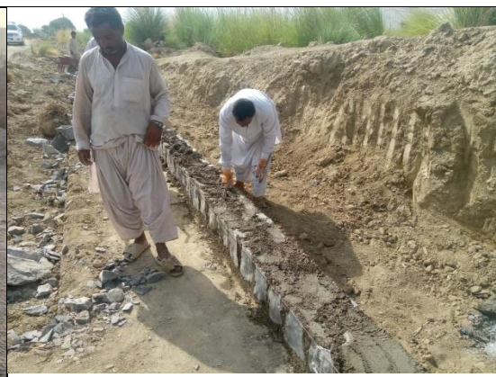
Workers not using proper PPE's.
