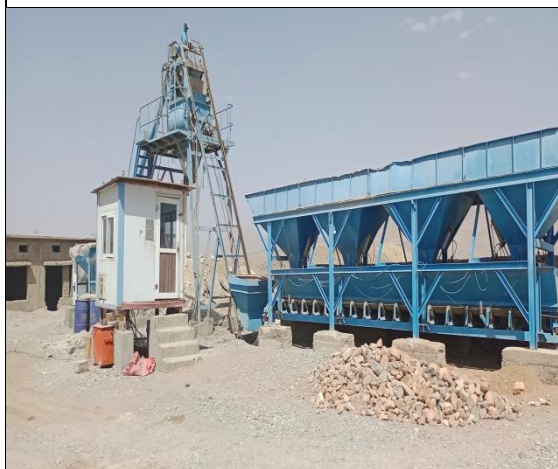
Warning tapes/sign boards not provided near crush plant.
