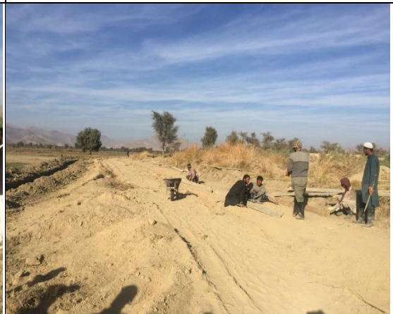
Workers working without proper PPE's
