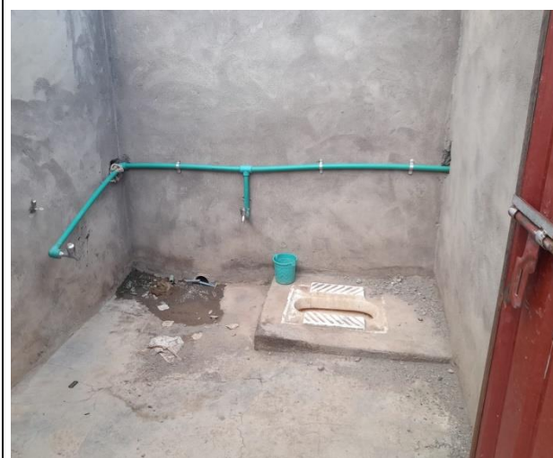
Workers washrooms in unhygienic condition
