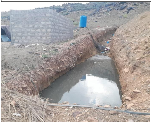
Improper wastewater disposal site near official residential rooms
