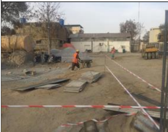
Warning tapes provided on site
