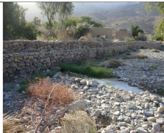
Hitachi Channel Required Rehabilitation
