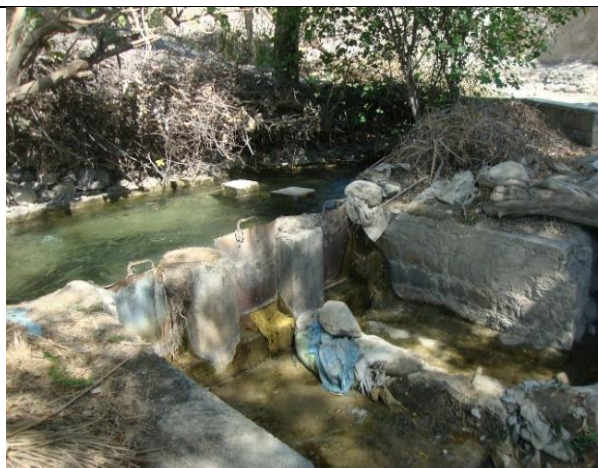
Hitachi Channel Required Rehabilitation
