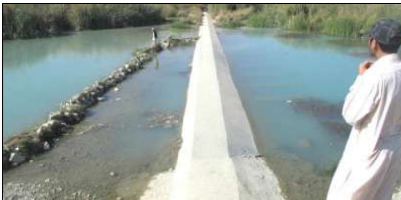
Figure 3: View of damage portion of Chutta Weir
