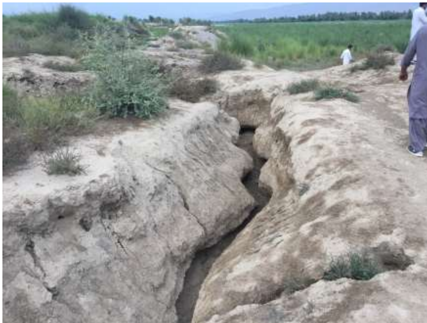
Figure 17: Erosion phenomena was observed on left bank of Chutta Weir
