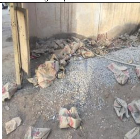
Empty cement bags are not properly disposed off
