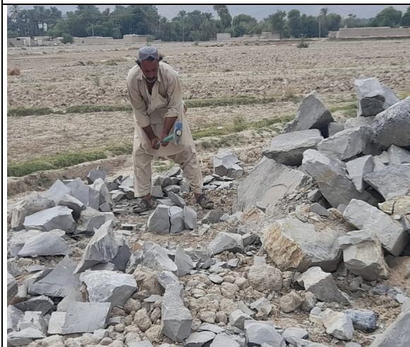
Worker working without using PPE's
