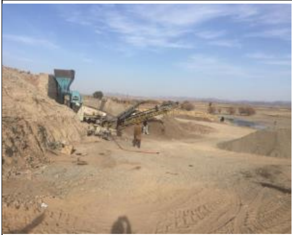
Warning tape or sign boards were not available
