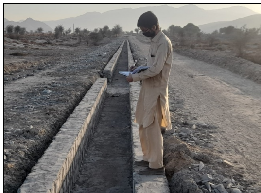
Construction of Chutta Right Sump No.1 in progress, water sprinkling greatly required
