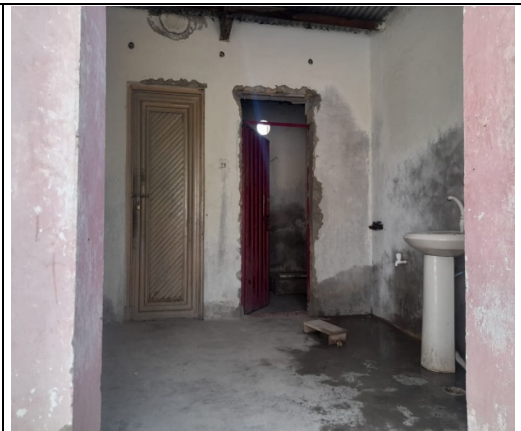
Proper hygienic washrooms are available for workers
