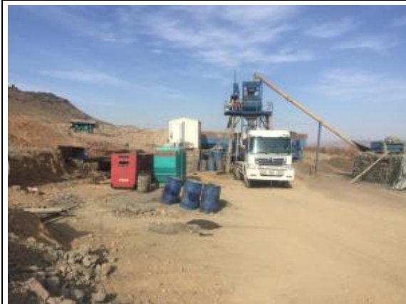
Leakage from generator
