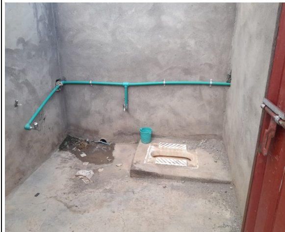
Workers washrooms in unhygienic condition
