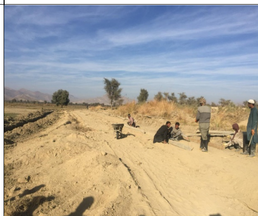
Workers working without proper PPE's
