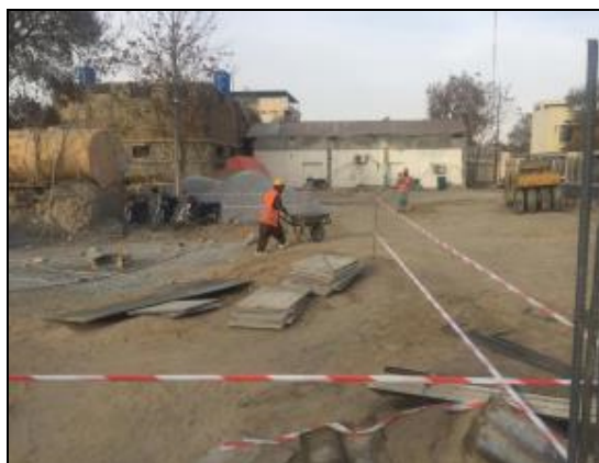
Warning tapes provided on site
