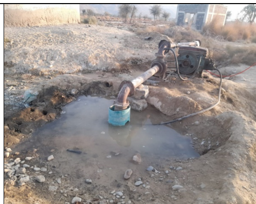
Chutta Left, Chutta Right and Chutta Main Sump No.1 distribution point
