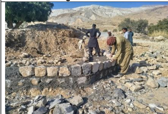
No PPEs Compliance
