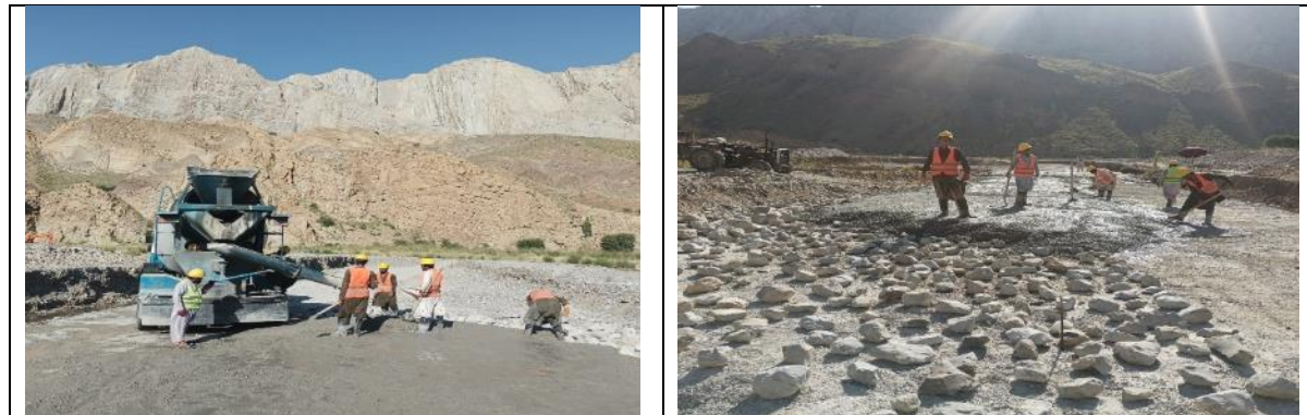
No Caution Tape and safety Sign Boards at Site
