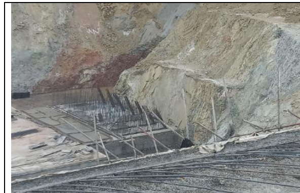
Sliding will be harmful for the workers
