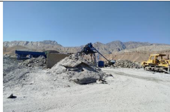
No safety signboards
