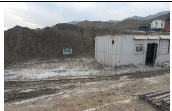
Lack of housekeeping on the dam site area, and the ground is observed uneven
