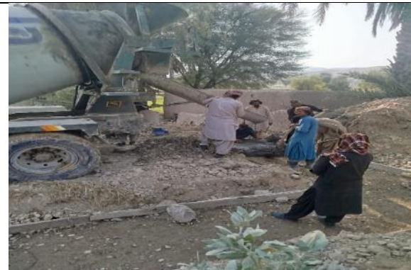
No PPEs Compliance
