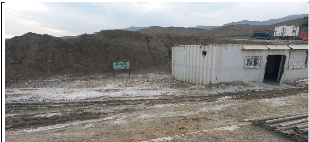
Lack of housekeeping on the dam site area, and the ground is observed uneven
