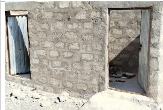
No cleaning of washrooms at site
