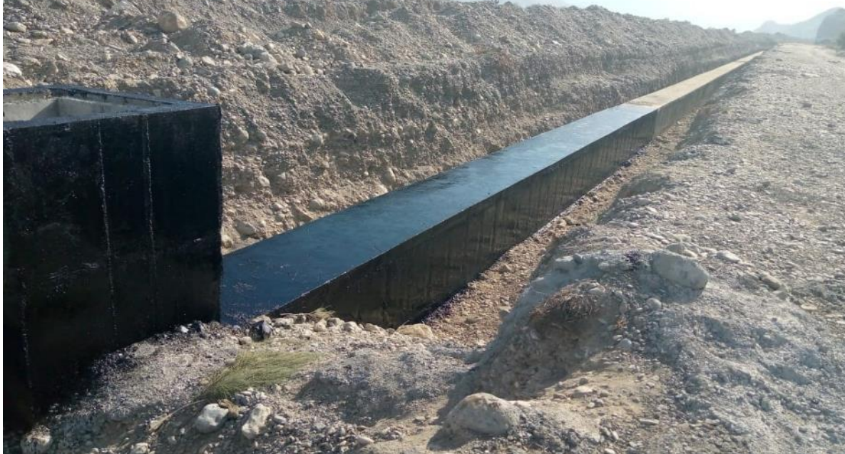
NCB-02 - Construction of Kharzan Hatachi Infiltration Gallery Subproject - Mula River Basin A View of Shajo Channel at Khrzan
