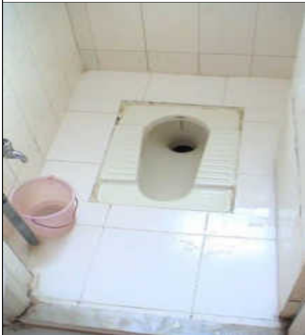
Hygienic conditions of workers washrooms
