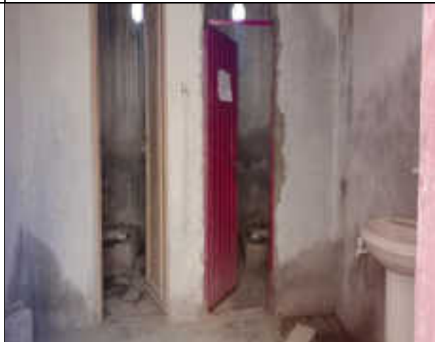
Washrooms in unhygienic conditions
