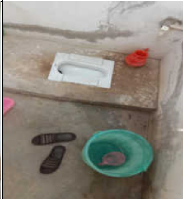
Washrooms condition changed after Non-compliance notices
