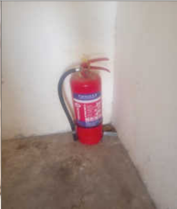
Availability of fire extinguisher at camp site
