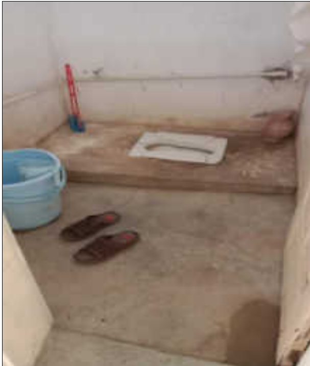
Hygienic condition of worker washrooms
