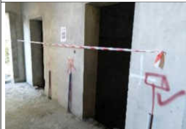
Elevator Shaft not barricaded Properly
