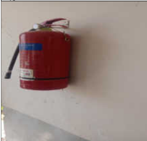
Fire extinguisher provided at camp site
