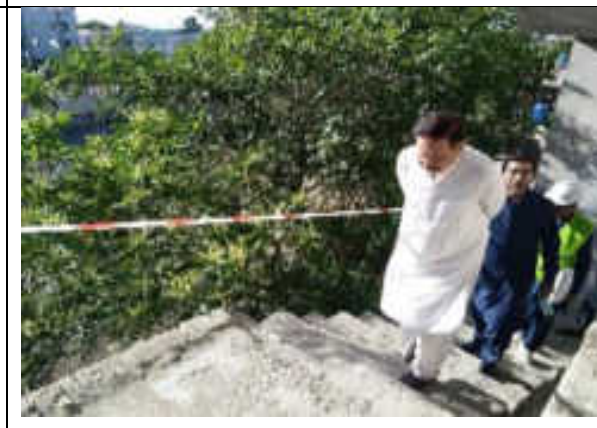
Elevator Shaft not barricaded Properly
